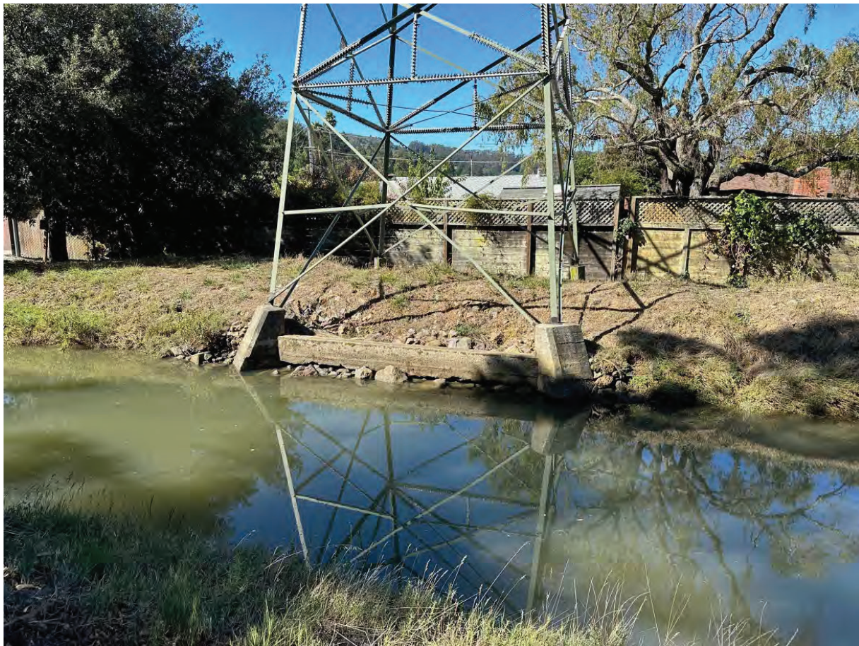
Photograph 1: Preconstruction Photo- Portions of the concrete footings of Tower 013/094 that extend into the mean high-water line of the channel, taken October 18, 2023, facing west.
