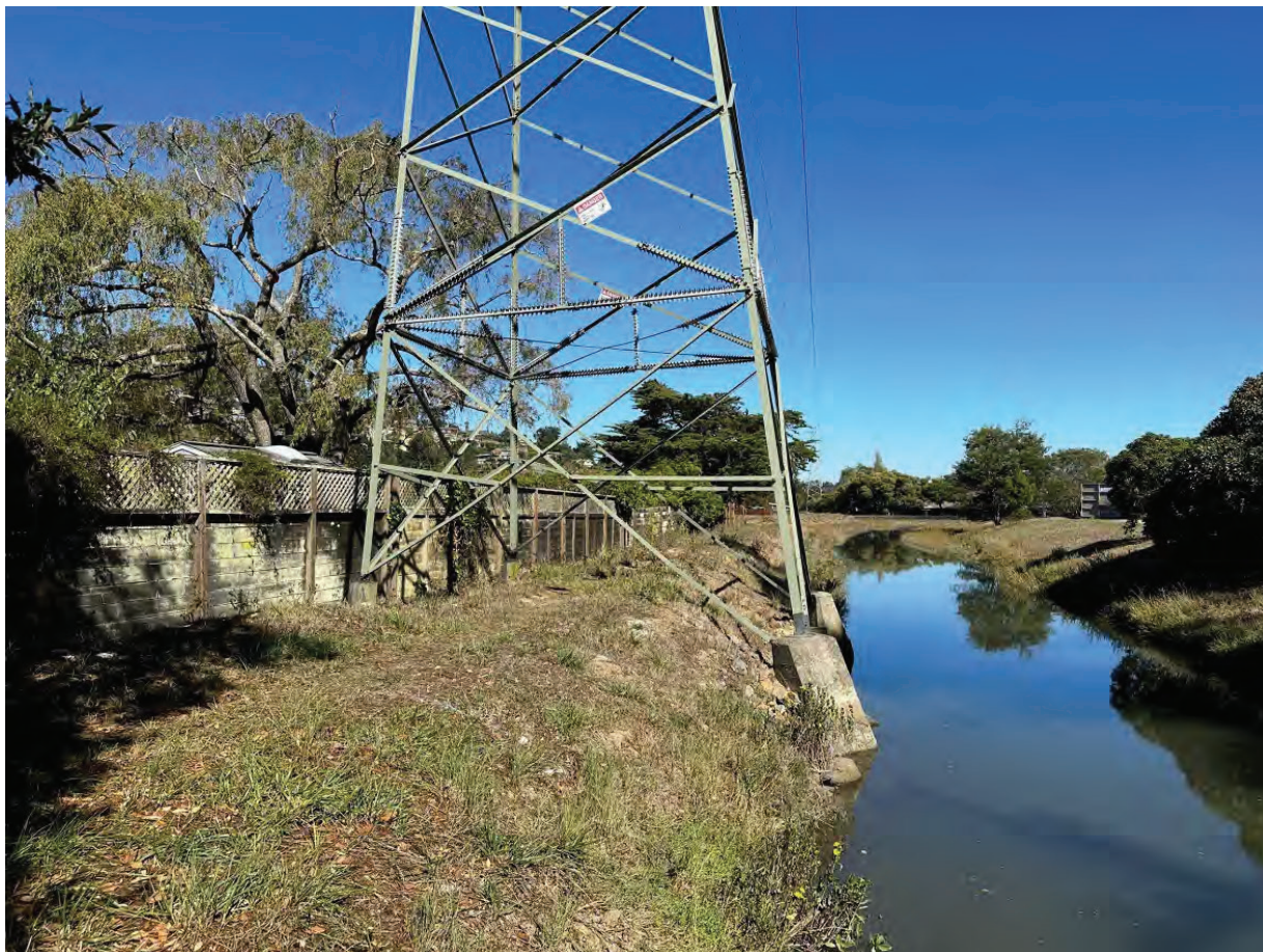
Photograph 2: Preconstruction Photo- Footings of existing Tower 013/094 with channel to the right looking downstream, taken October 18, 2023, facing north.
